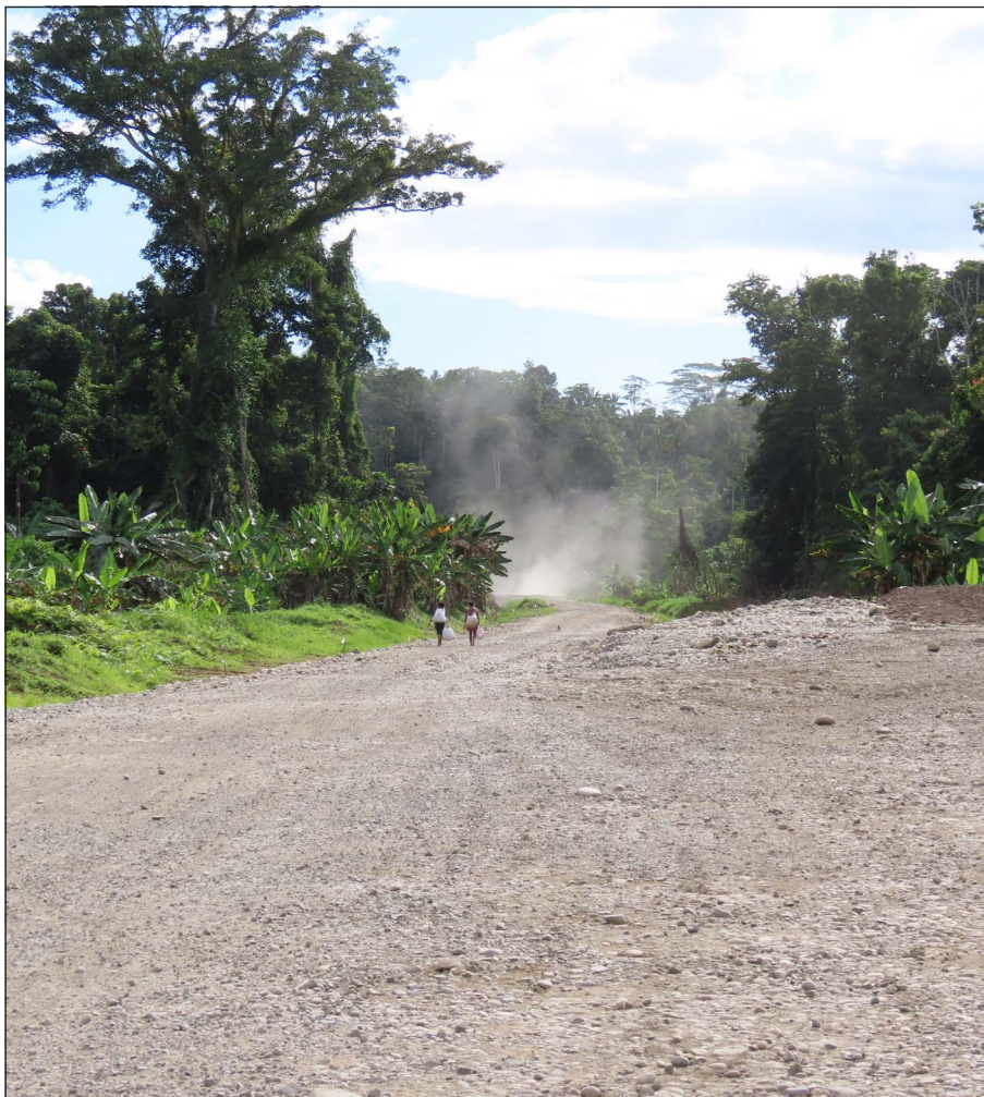
Plate 9.11 ITCS Road construction dust
