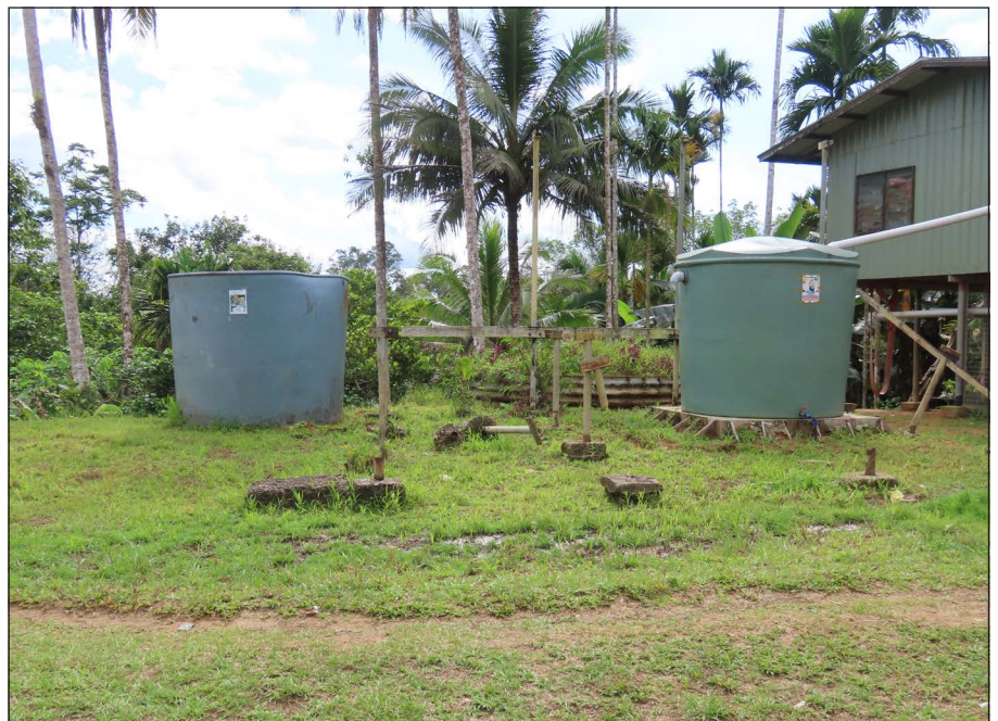
Plate 9.28 Rainwater tanks, Birimkamba village
