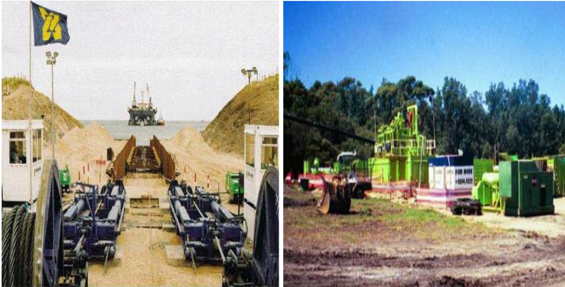
Figure I-13 Near Shore Pipeline Installation Method (Shore Approach): Shore Pull Trenching (left) and HDD (right)
