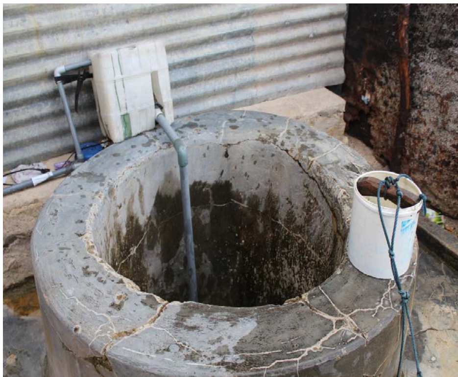
Figure II-245 Well in Sisir Village, Kokas District
