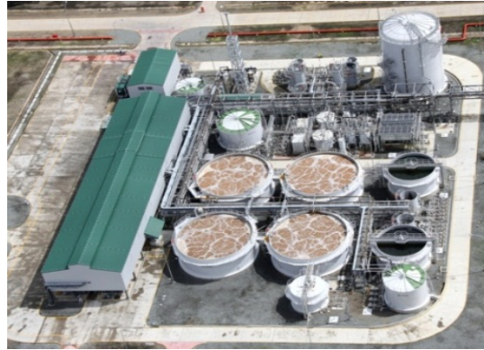
Figure I-3 Existing Produced Water Treatment Unit at Tangguh LNG
