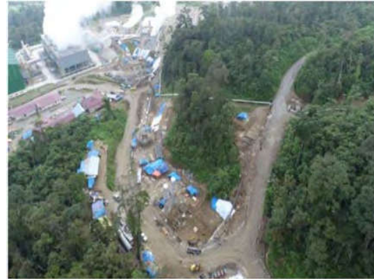
Silica Scaling Mitigating Facility
