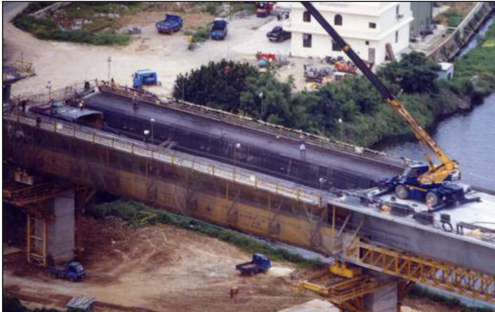
Figure 8: MSS in Place Awaiting in Situ Construction, Taiwan High-Speed Rail, ROC (Photo courtesy of THSRC)
