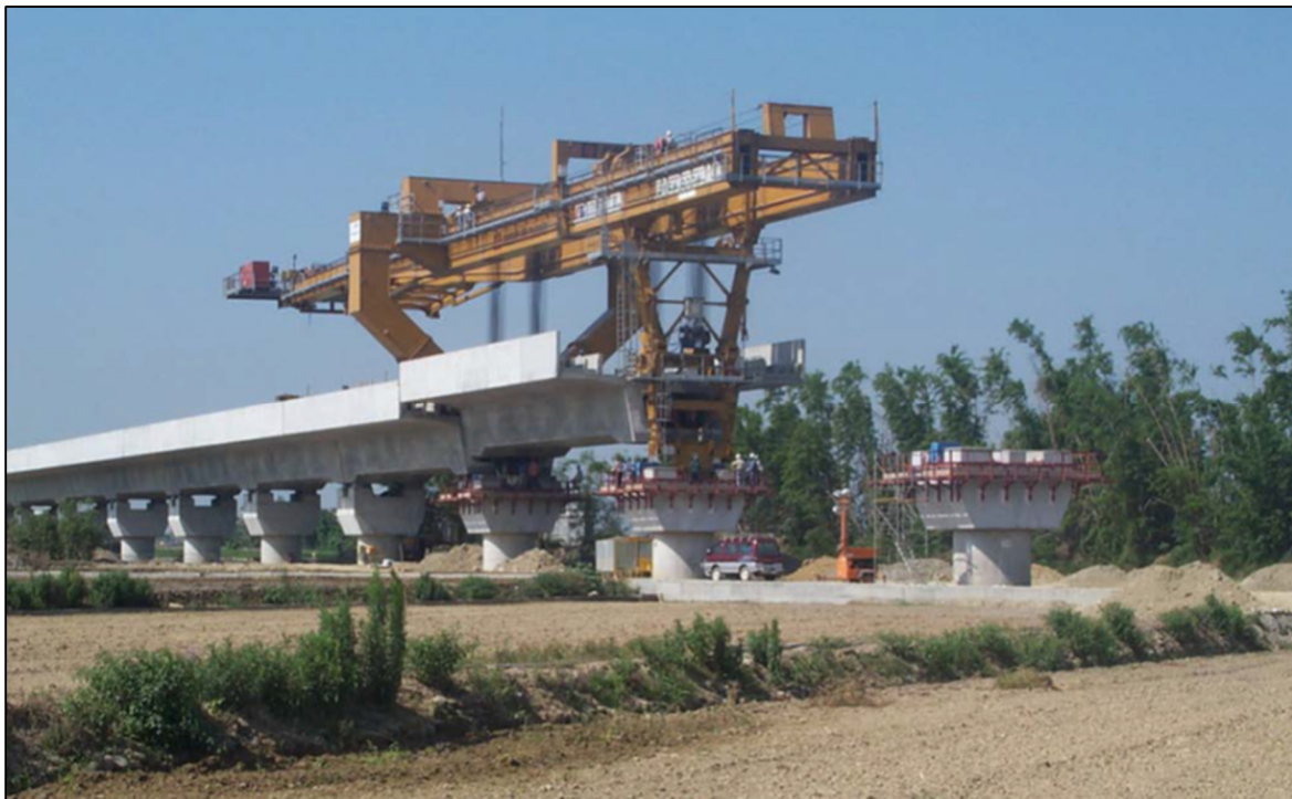
Figure 5: Launching/High-Speed Rail System under Construction in Taiwan, ROC (Photo courtesy of THSRC)
