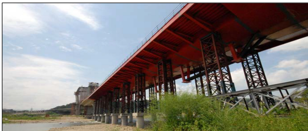
Figure 3: Staging and Falsework Supporting the Formwork for In Situ Construction ( Photo courtesy of Taiwan High-Speed Rail Corporation [THSRC] )
