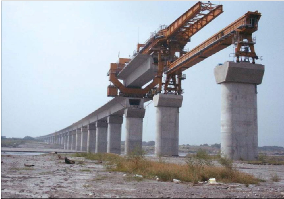
Figure 6: The Full-Span Precast Launching Method Launching/High-Speed Rail under Construction in Taiwan, ROC (Photo courtesy of THSRC)
