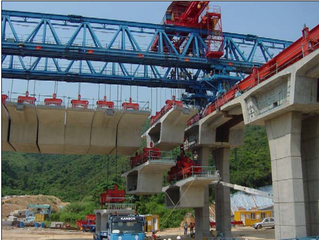
Figure 2: Deep Bay Link Bridge in Hong Kong, Precast Segmental Span-by-Span Method Using Overhead Gantry
