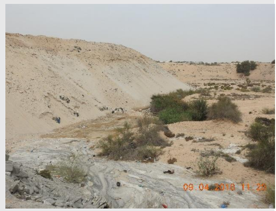
Photo B – Surface Water Body, Suspected Leachate, at Toe of Slope of Solid Waste Landfill Area (not within Project's construction limits of disturbance)
