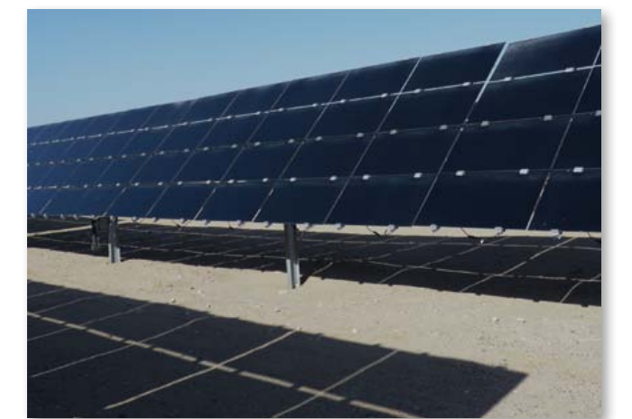
Panels, which change the angle in accordance with the sunshine angle, are always kept clean.
