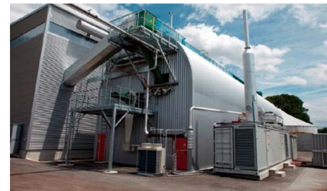
The same plant as the waste treatment and power generation plant of the California project
