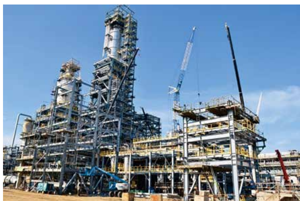
Polyethylene manufacturing plant
