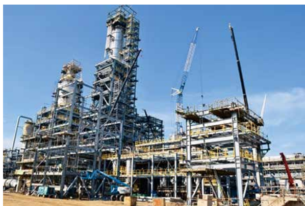
Polyethylene manufacturing plant
