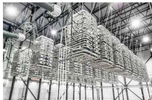
High Voltage Direct Current Offshore Electricity Transmission System
