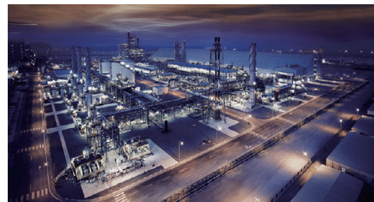
An ammonia production plant under construction in Al Ruwais, Abu Dhabi, which is scheduled to begin producing clean green ammonia by 2030. (Photo provided by MITSUI)
