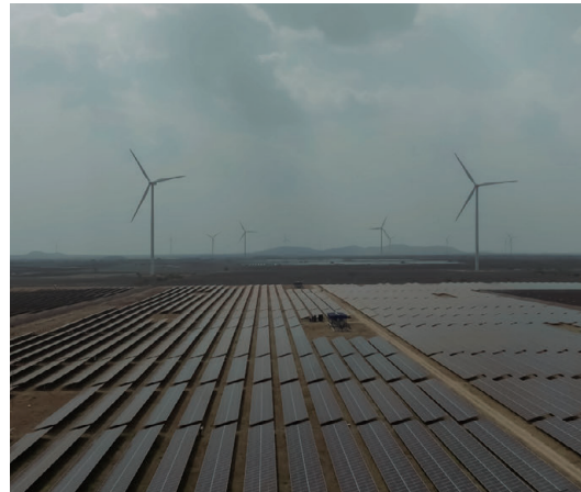
Renewable energy facilities currently operated by CleanMax. The electricity generated contributes to the decarbonization efforts of its customers. (photo provided by Osaka Gas)
