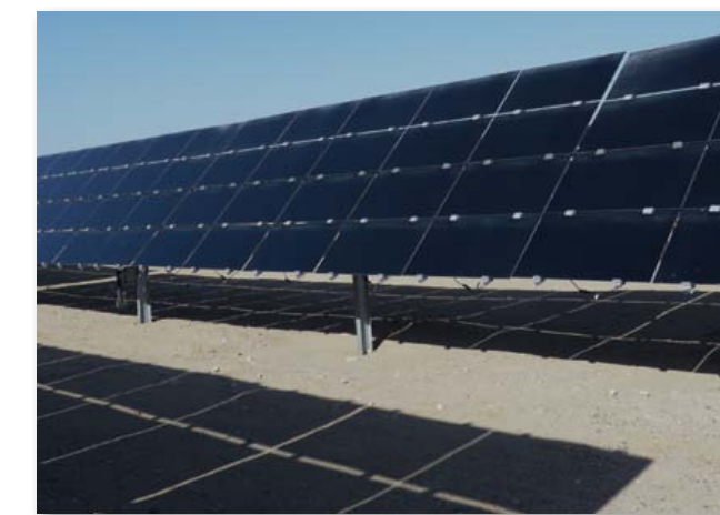
Panels, which change the angle in accordance with the sunshine angle, are always kept clean.
