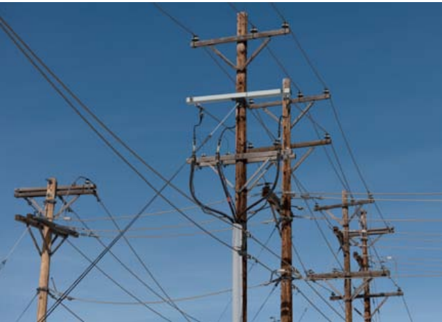
U.S.: Rapidly aging electric power cables
