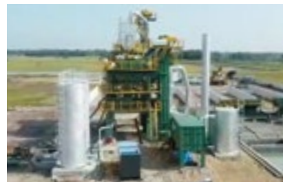
No.2 recycled asphalt plant built in Majalengka City, Indonesia
