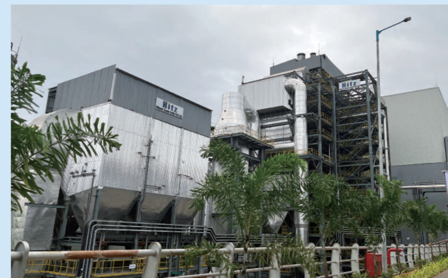
Power generation using waste has been used throughout Japan since its high-growth period of the 1960s. The spread of Japanese technologies is expected to contribute to solving India's economic and social infrastructure challenges.
