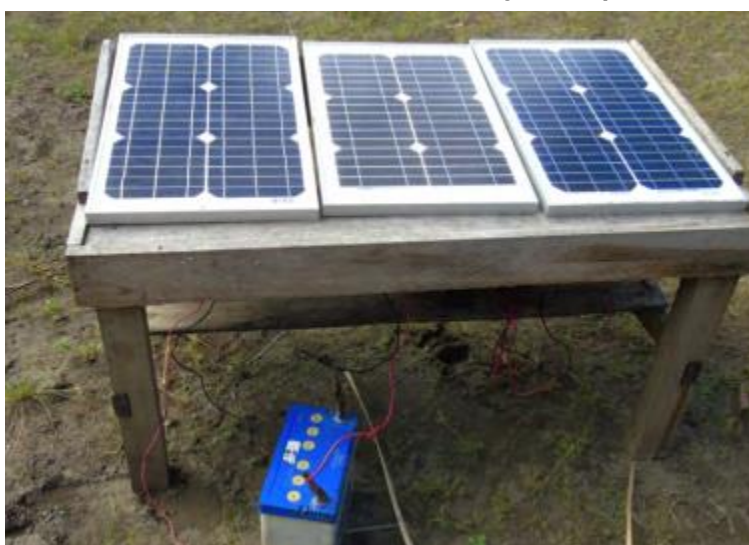
Plate 9.6 – Solar Panels and Battery at Maipenairu
