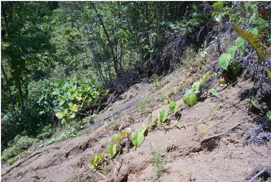
Plate 8-7 Landslip on an Antelope 3 sidecast slope showing failed rehabilitation
