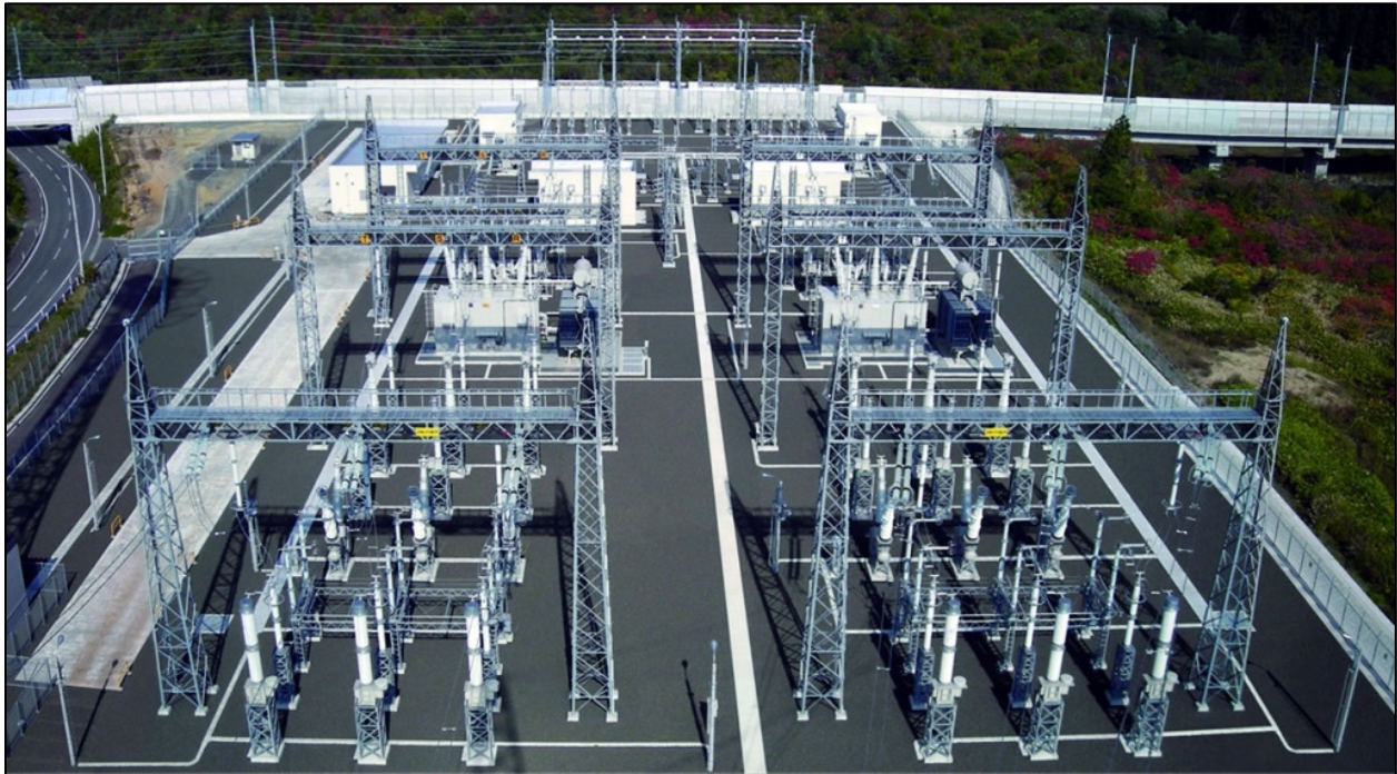
Figure 2-15: Typical HSR TPSS
